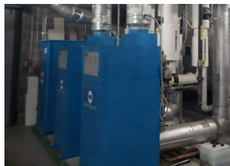
Heating Water Boilers
