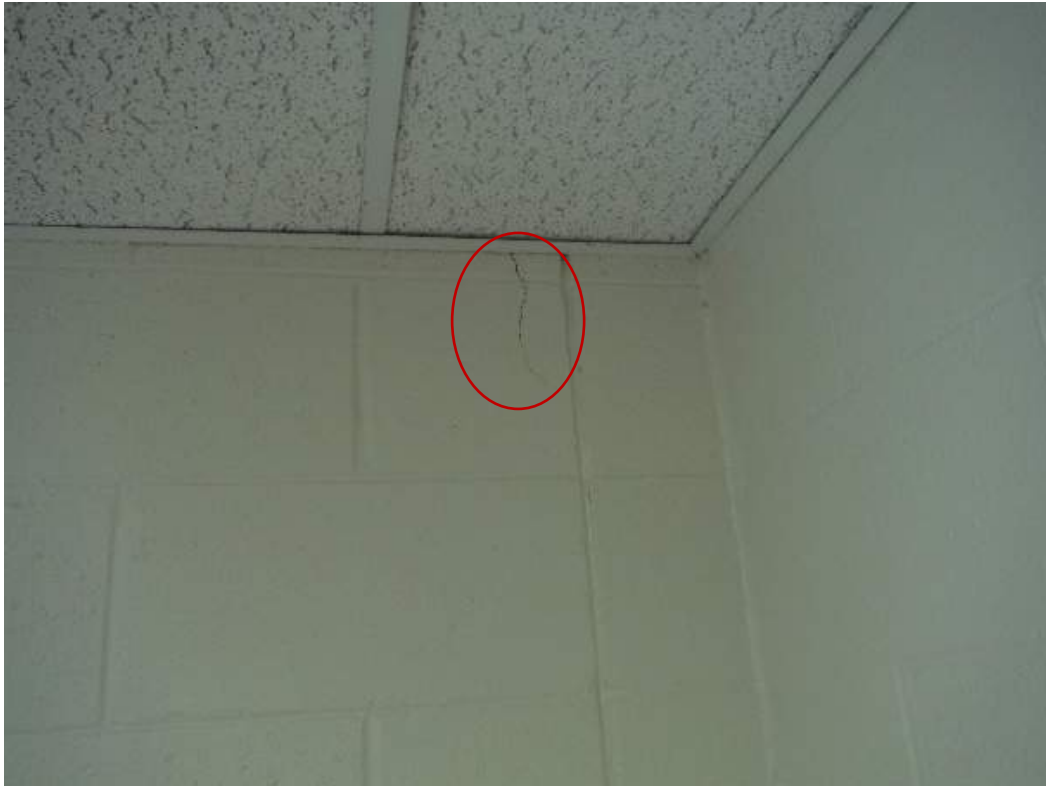
Area C - Cracking in Exterior CMU Wall South of Range
