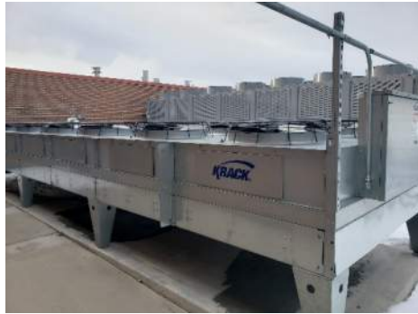
Fluid Cooler & Chiller
