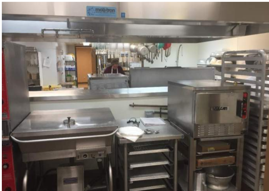
Kitchen is Full of Cooking and Preparation Equipment
