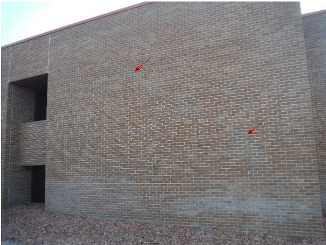
Area A – Repaired Cracks at North Wall
