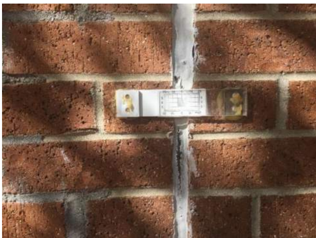
Building Joint Caulking Brittle and Cracking
