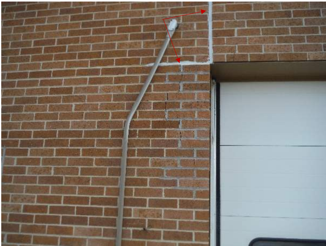
Area C - Repaired & Unrepaired Cracks at Maintenance Door
