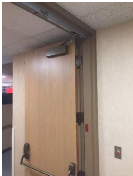
Door in 2 HR Assembly w/ MHO Release
