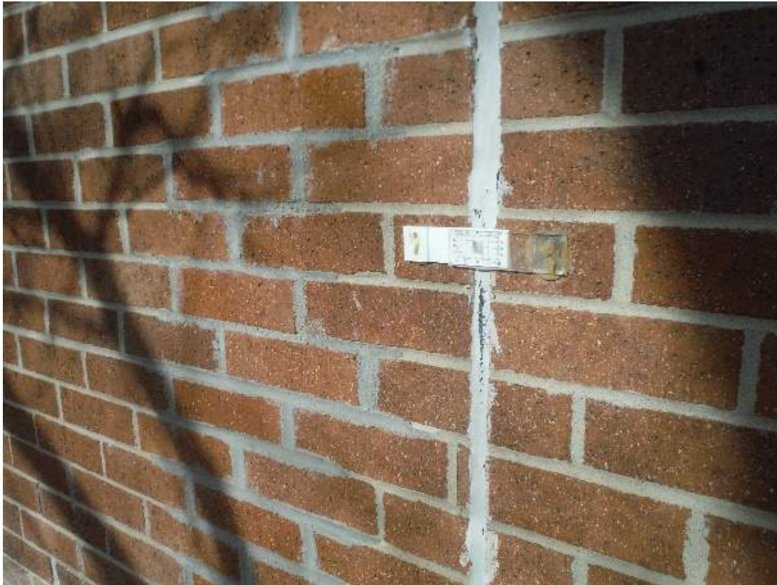
Crack Gage at CMU Control Joint at South Wall of Fire Range
