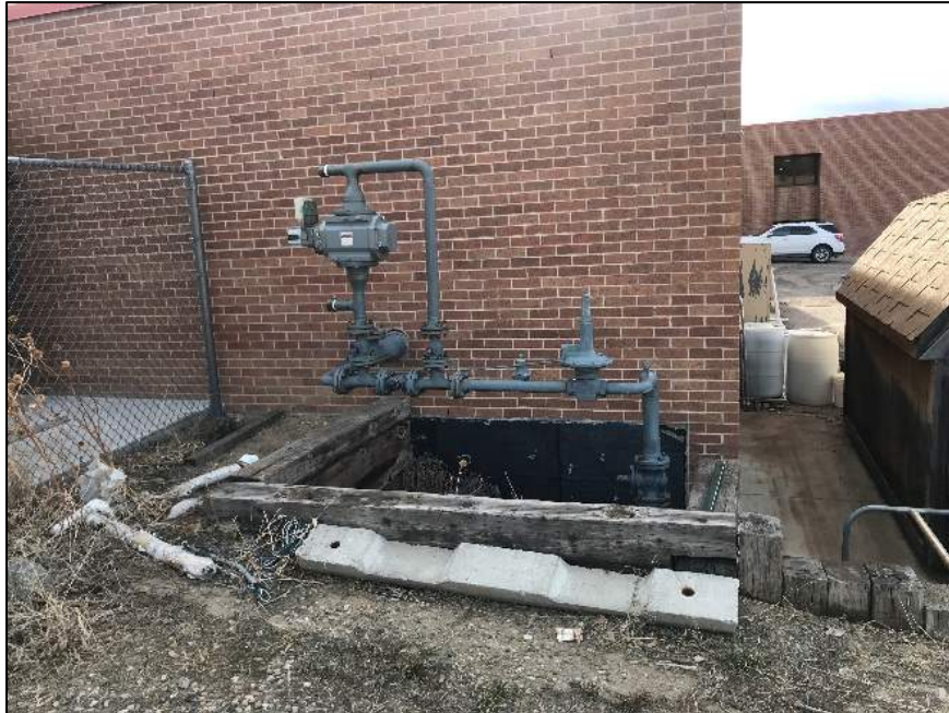
Gas Meter at Northwest Corner Near Mechanical Equipment
